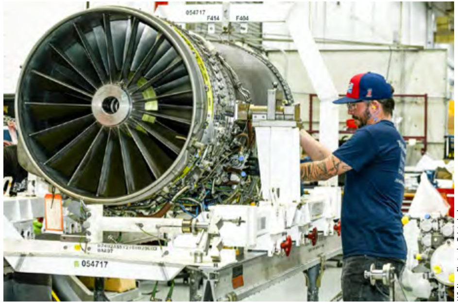
Aircraft Mechanic Michael Pucket installs a fan geometry actuator on an F414 engine.
